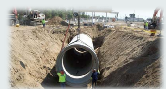
Figure 2 Storm water sewer [2]
